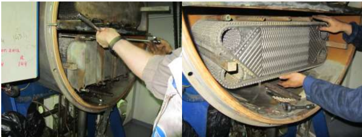
Figure 8. System is opened and cover is removed. Water released is clear.
