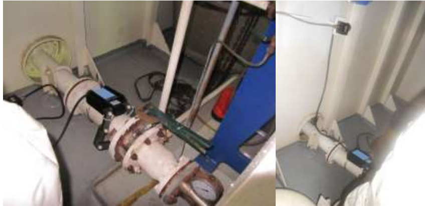
Figure 6. Left: System experimental installation location. Right: System is connected to an EJB connection.
