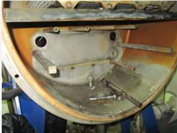
Figure 12. June 2013 – FWG chamber (where plates are mounted) treated with HydroPath MARINE technology without any limescale or slime.
