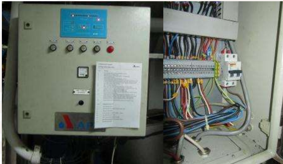
Figure 7. FWG main power cabinet and cable connection
