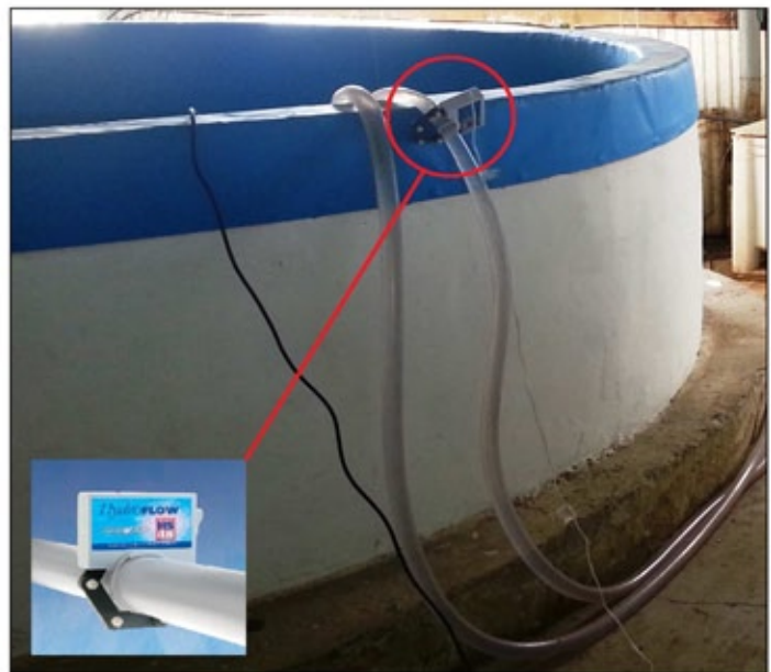
Installation of the HYDROFLOW system on the water inlet to tank # IV
